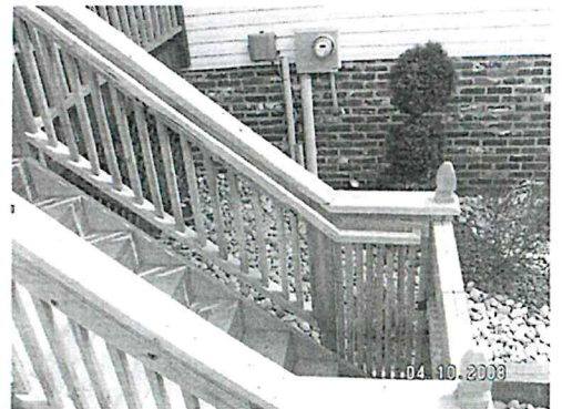
Figure 6. Release mechanism located 3" (min) down from top, inside of gate at bottom of stairs (photo is showing 12" from the top). Safety barrier with maximum 1/2" openings is within 18" of all directions of the release.
